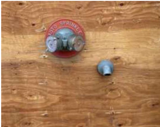
ATB Fire Department Connection
