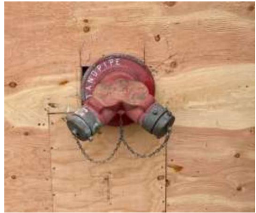
FSS Tower Fire Department Connection
