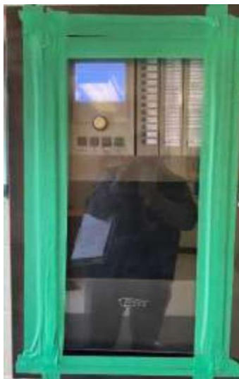
FACP in South Lobby
