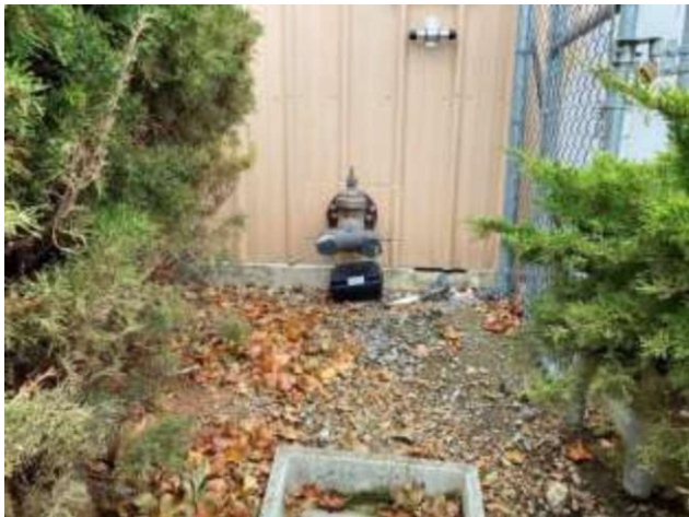
Fire Pump Test Header
