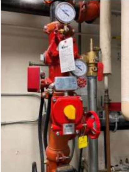
Sprinkler Control Valve
