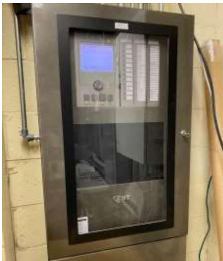
FACP in Electrical Room
