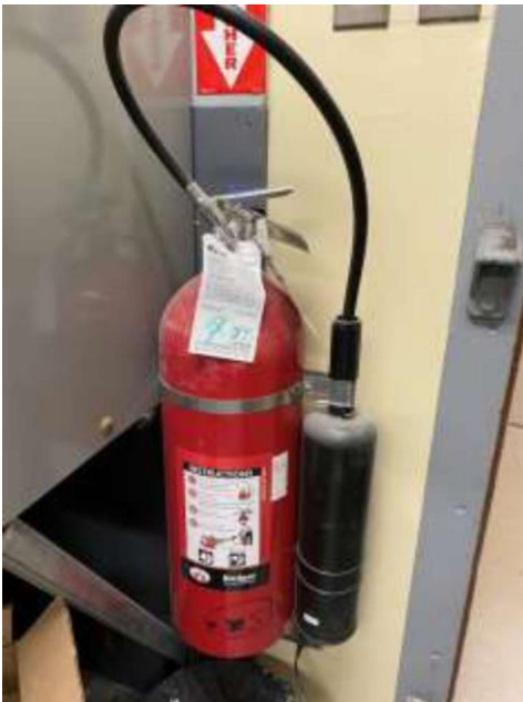
Carbon Dioxide Extinguisher
