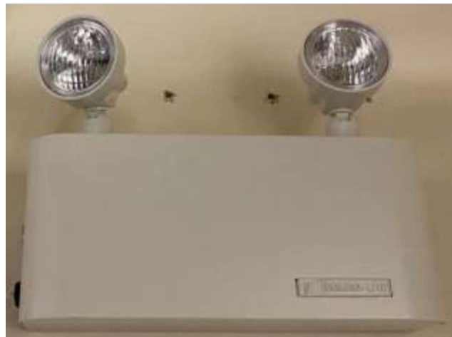
Battery Pack & Lights
