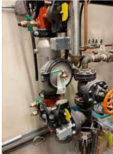
Main Valve & Backflow Preventor
