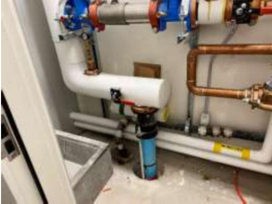
Northwest Water Entry Room
