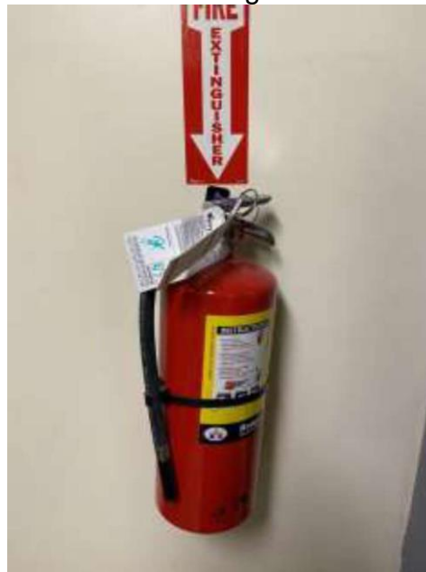
Dry Chemical Extinguisher
