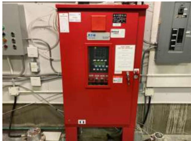
Fire Pump Controller
