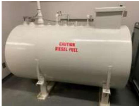
Generator Fuel Tank
